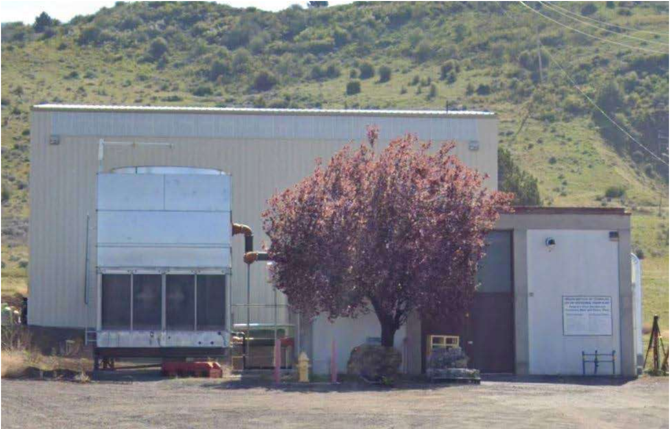
Large Geothermal Power Plant
