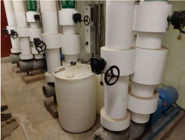
Secondary Chilled Water Pumps
