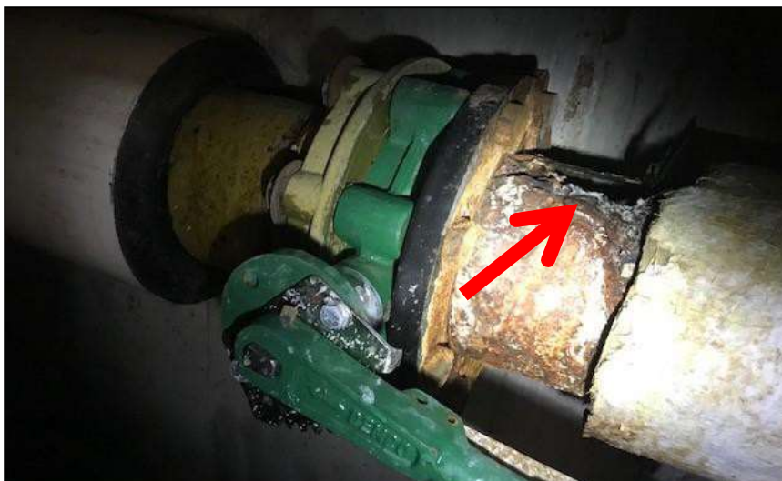
FIGURE 4: RUPTURED PIPE IN TUNNEL
