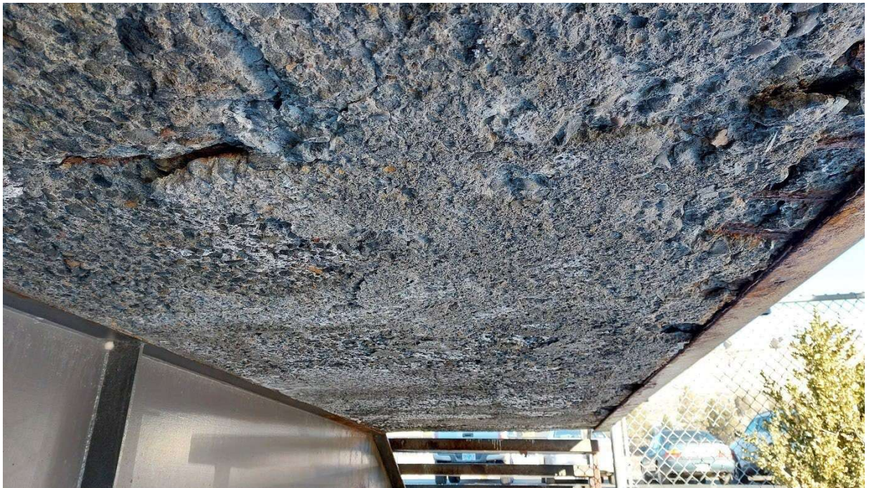
Figure 2: Concrete Deterioration at underside, exposing rebar
