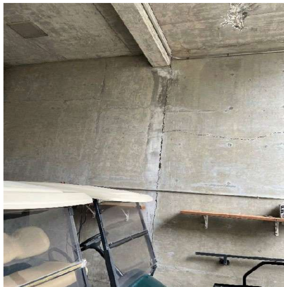
Figure 3: Retaining Wall Vertical Crack
