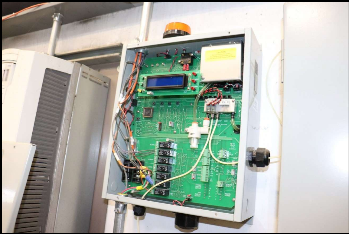
Figure 9 Control box with cover removed
