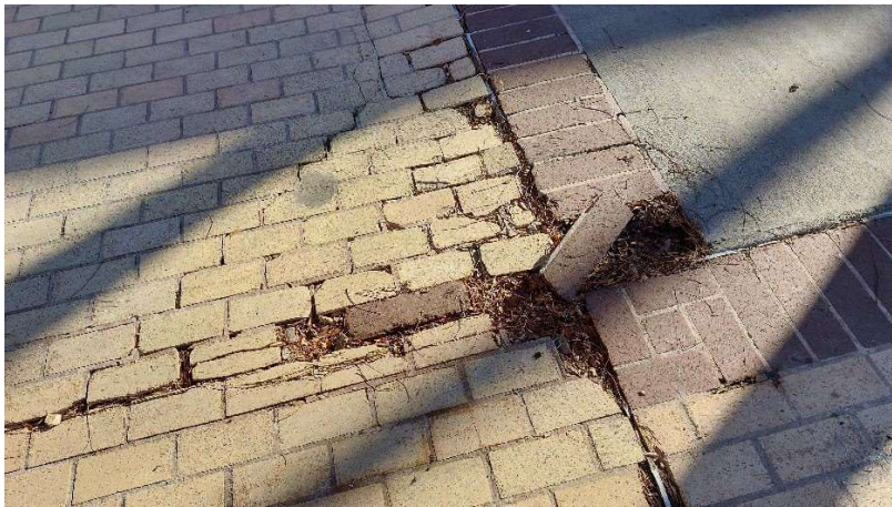
Broken brick paving
