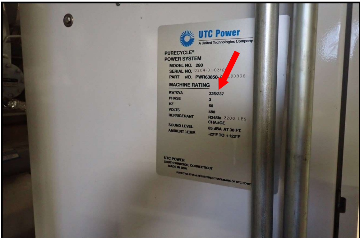
Figure 14 Plant C label plate, arrow points to rating of 225 kW
