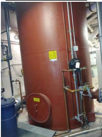
Condenser water tank
