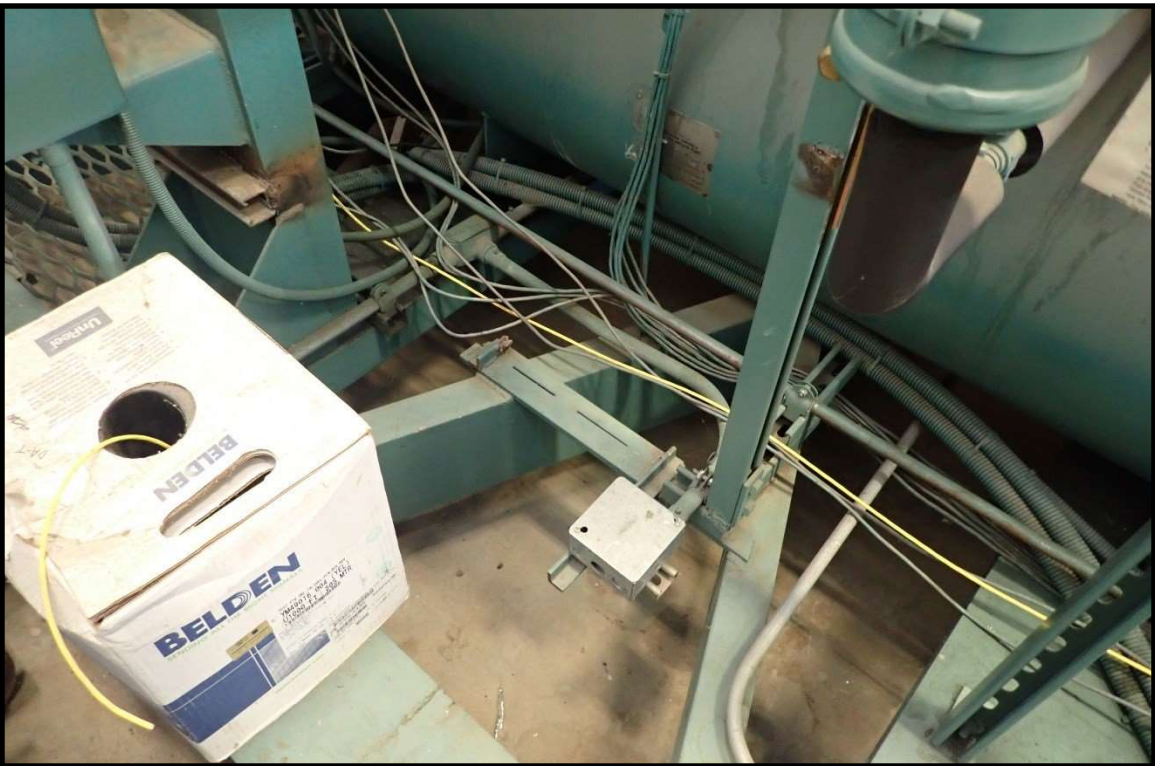
Figure 8 Alternate view of ORPP showing wires not in conduit and strewn about haphazardly
