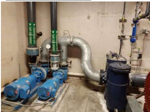
Condenser Water Pumps
