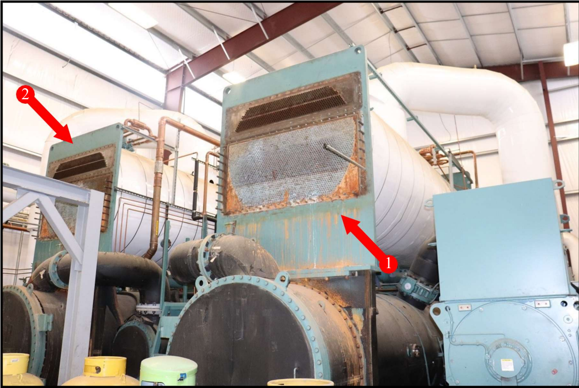
Figure 1 Inside the ORPP building showing partly disassembled system Arrow 1: Plant A Arrow 2: Plant B
