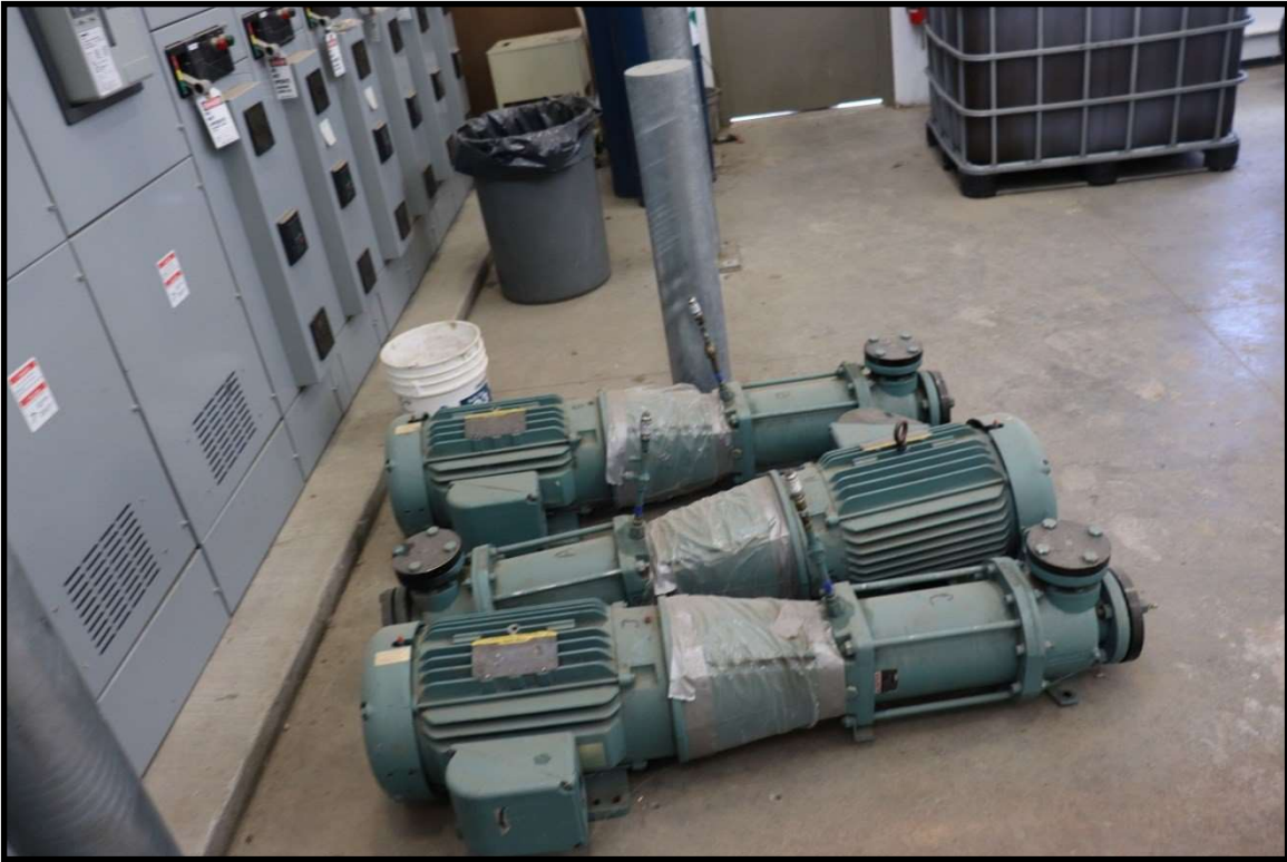
Figure 3 Feed pumps not installed
