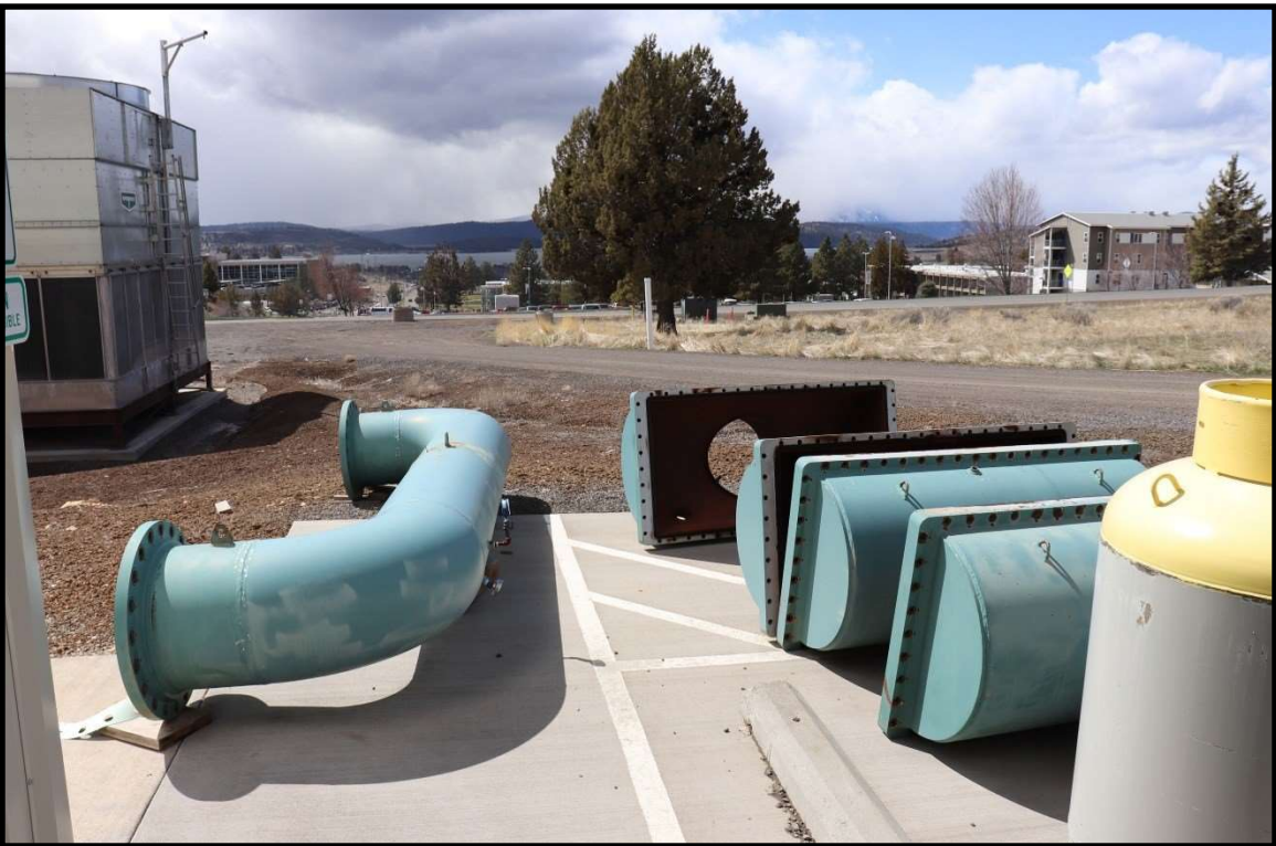
Figure 4 View outside the ORPP building showing covers and piping removed from system
