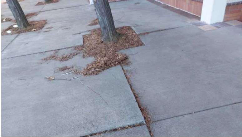
Frost heaves at slabs
