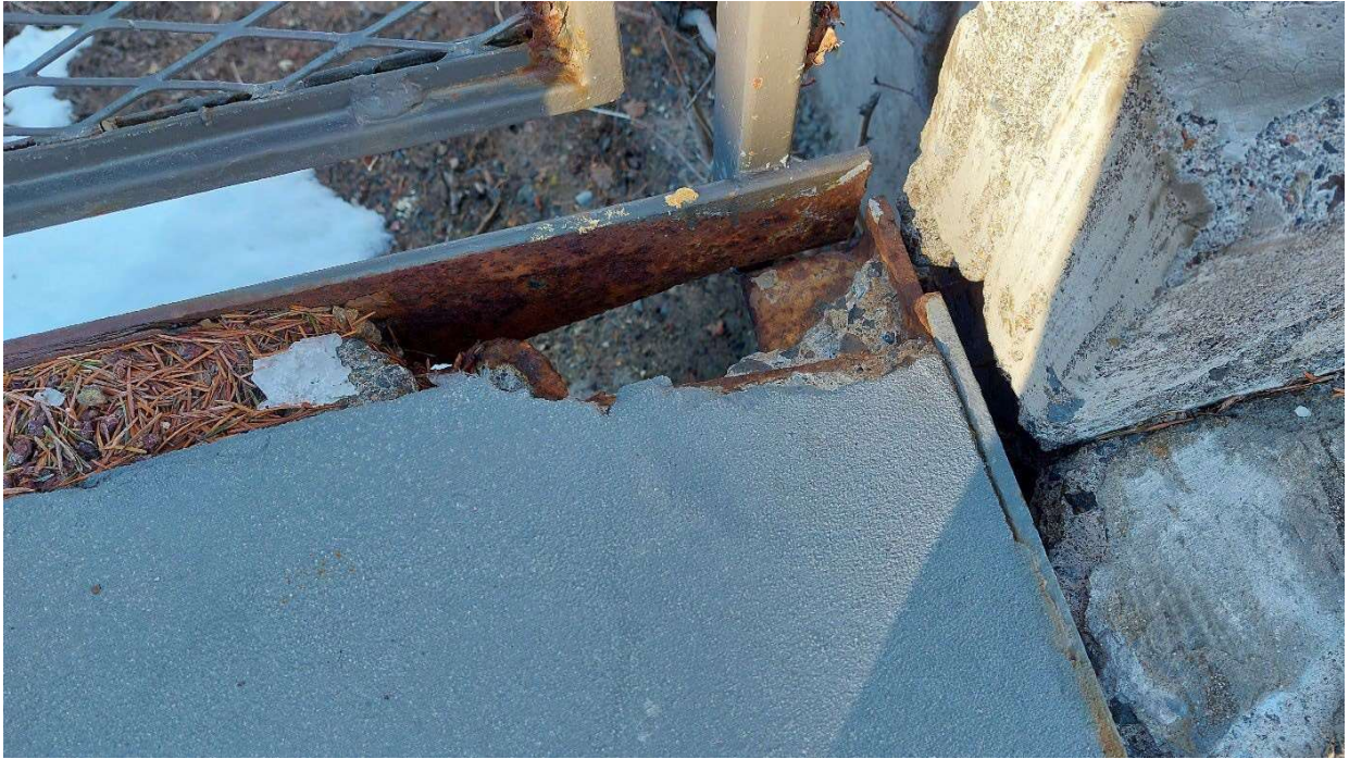
Figure 1: Bridge Corrosion at top surface
